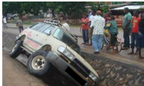
Dangerous deep open drain parallel to road
